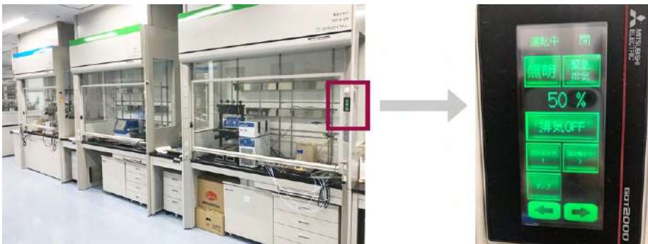
Low air volume (push/pull type), ultrahigh speed variable air volume (VAV) local ventilation device (exhaust fan output visualized on the operation panel) (Minase Research Institute)
