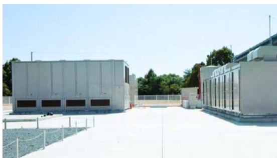
Large-capacity power storage system (Yamaguchi Plant)
