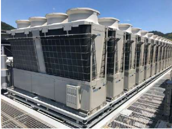
Module-type heat pump chiller (Minase Research Institute)
