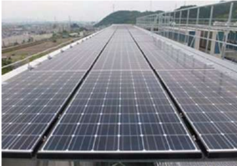
Solar panels (Minase Research Institute)
